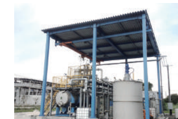
Recycling equipment installed in the Kitakyushu Plant
